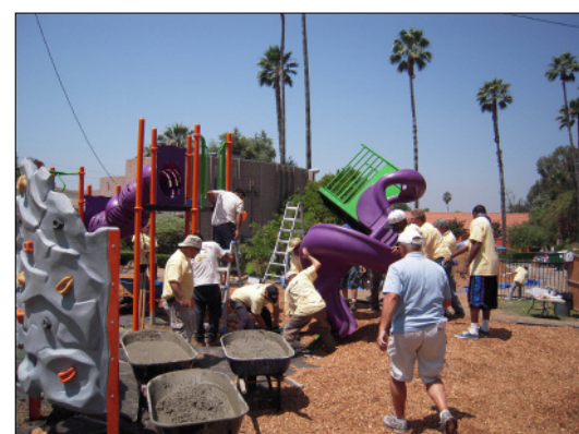
More volunteers team up to lift the "slide" portion of the playground set into place as wheelbarrows of "ready to pour" concrete are lined up and ready to go.
